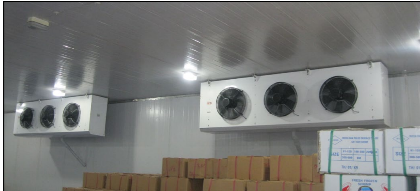
-20 °C cold room
